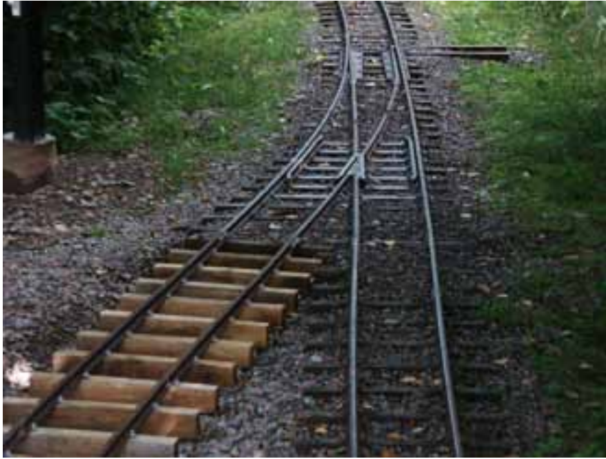
Figure 2b: Construction of passing loop showing several elements of track construction. With the stake pins of the foregoing figure providing reference, the track is removed and a shallow ditch in the track position dug, so the track can be sunk into the bank. Only then the second rail is attached. The photo shows the new track in this situation, before the final filling of ballast. A fiber cloth is present at the bottom of the ditch but cannot be seen in the photo. The new point has not yet been provided with its throw mechanism.
