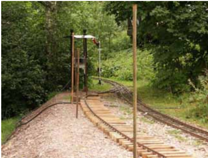
Figure 2a: Construction of passing loop showing several elements of track construction. Before laying into place, the track is preassembled with only one rail attached. It is thus still highly flexible and can be sprung to its proper location (with the proper bends) and weighted down with stones as required. Reference stake pins are then located at some offset besides the track. In the picture, also note stop signal showing clear and signal box for driver control of signals.
